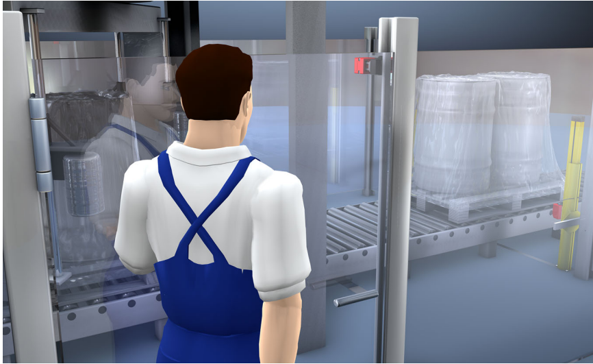
S200 Safety Switch on the door of a plastic film wrapping station
